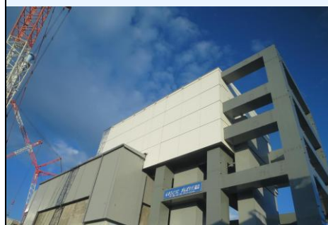
Removal of Fuel from the Spent-Fuel Pool of Reactor 4 – Fukushima Daiichi NPP, Japan – December 2013
